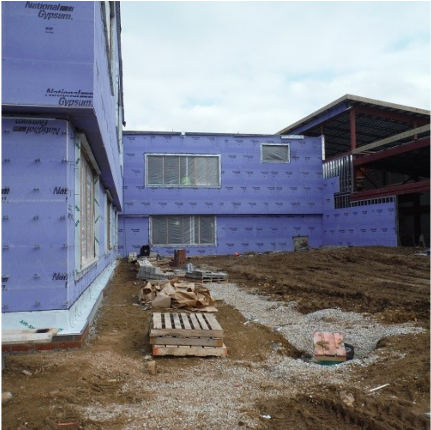
Photo 2 shows fiberglass-faced gypsum-board sheathing over steel stud framing, which will be covered by brick or stone masonry or decorative metal panels.
