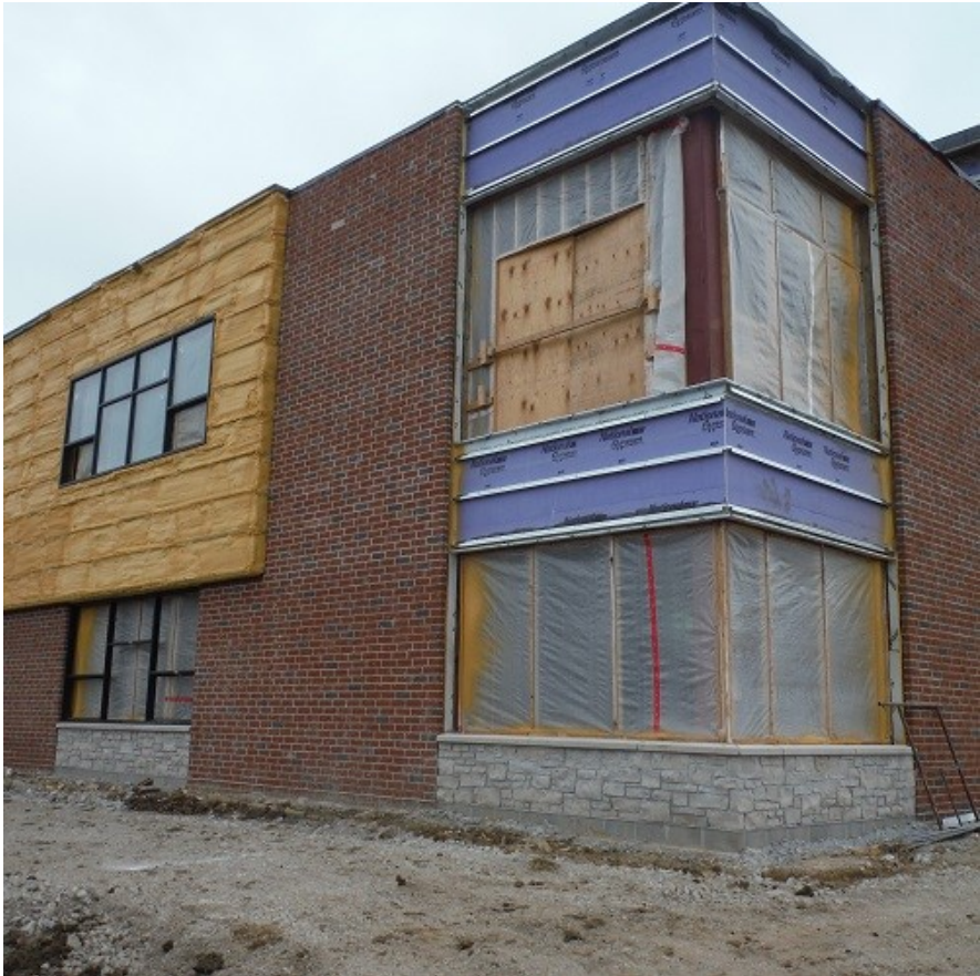
Photo 3 shows the finished masonry, ready for the installation of decorative metal panels.
