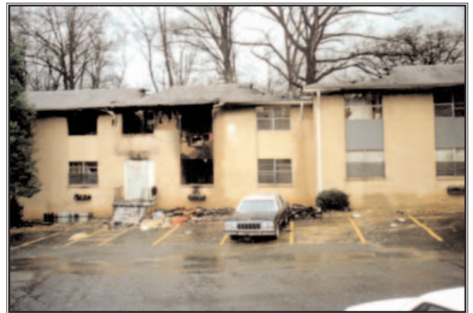
Fire station within 300 yards. Response time 2 minutes. Eight families homeless
