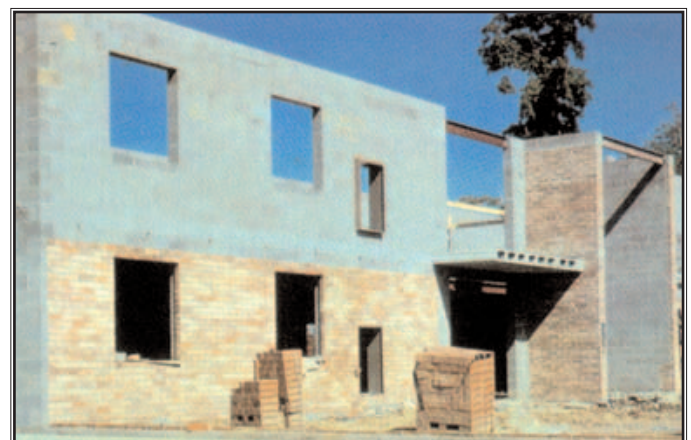
These concrete and masonry residential buildings cannot add fuel to a fire, and will confine fire to the area of origin
