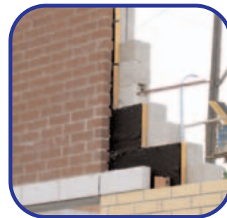
New Berwyn Middle School Architect: Green Associates, Inc. - Deerfield, IL Mason Contractor : Piazza Masonry - Lockport, IL
