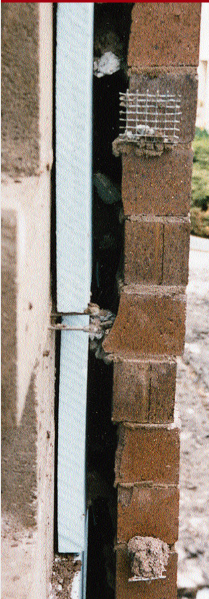
The mortar bridging and impaction in this 2-inch airspace are unacceptable.
