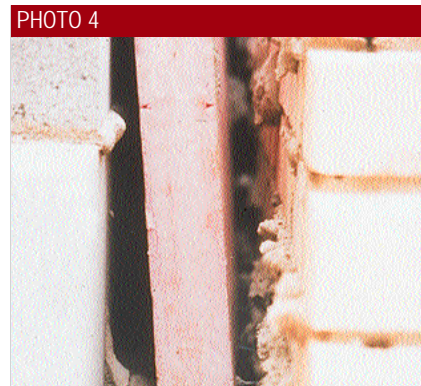
Misaligned rigid board insulation exposes this airspace to water bridging.
