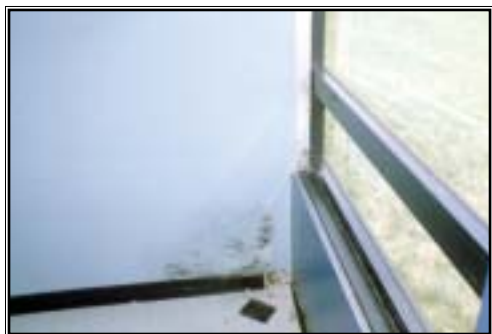
Notice the mold growing on the drywall near the floor.
