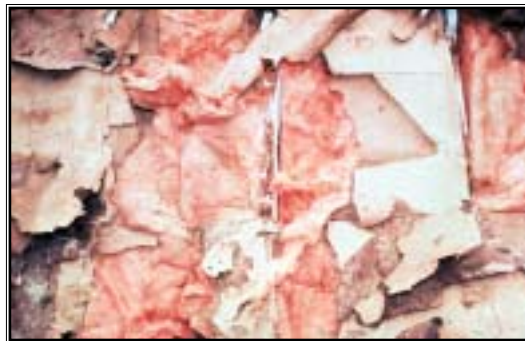
After the brick was removed one can see the corrosion of the steel studs, a black mold growing on the exterior paper of the drywall and saturated batt insulation at the base of the wall.
