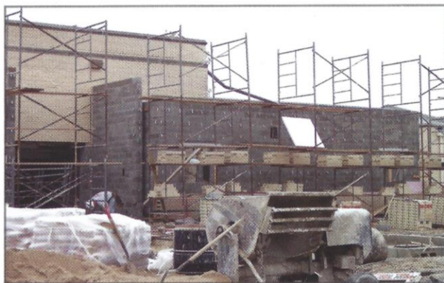
This project addition in the western suburbs used corrugated ties and had other major masonry problems. It has since been torn down and will be rebuilt in the spring.
