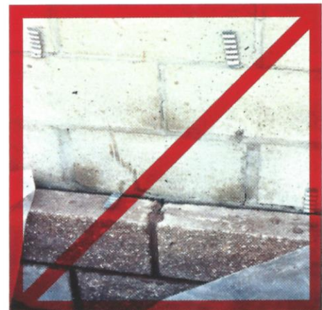
In this example, the use of corrugated ties in a brick / block cavity wall is illegal and not built to code!
