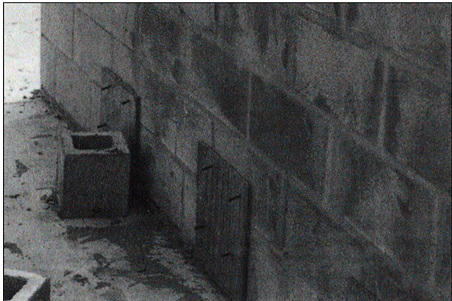
High-lift grouting requires cleanout openings to allow removal of debris from the bottom of each reinforced vertical core. Before grouting, the openings are covered with plywood forms.
