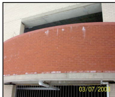
Local Hospital (Houston Architect): (Note the efflorescence and the flush cap- should have had 1 1/2" projection with drip edge, and flashing under cap.)
