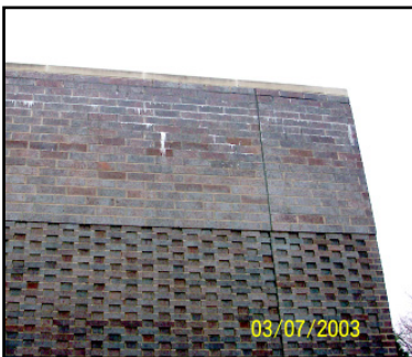
My Bank: (Note the efflorescence, and the flush limestone cap- it should have had 1 1/2" projection, with drip edge and flashing under the cap)
