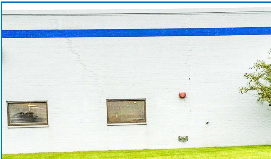
This older painted clay brick wall is showing signs of settlement and lacks properly located expansion joints.
