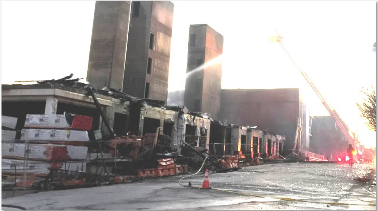
Concrete block stair and elevators outlasted the fire. Concrete block do not burn!
