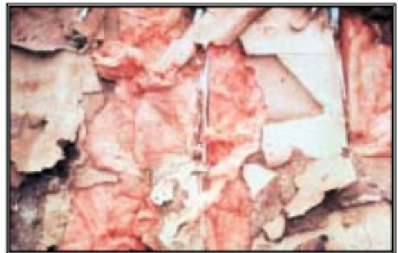
After the brick was removed one can see the corrosion of the steel studs, a black mold growing on the exterior paper of the drywall and saturated batt insulation at the base of the wall.
